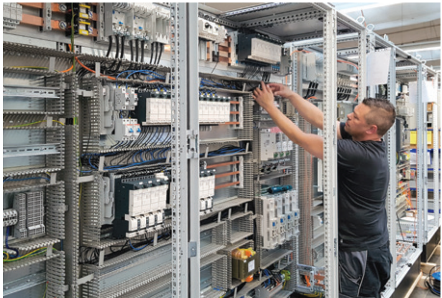
The often multiple-field switch cabinets are constructed in-house at BSG, wired, tested and shipped worldwide.
